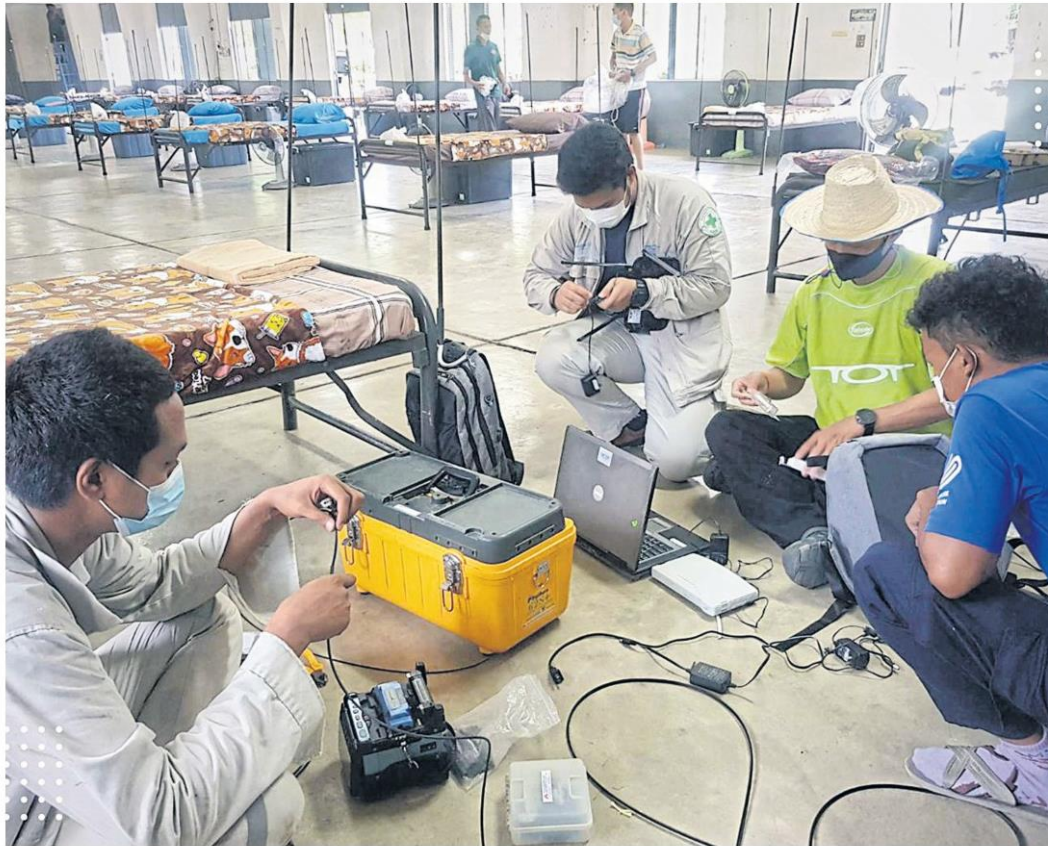
National Telecom has installed WiFi and IP Phone systems as well as CCTV cameras at field hospitals catering to Covid-19 patients.
