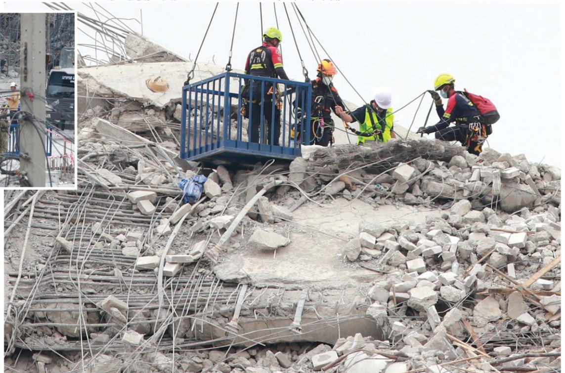
Rescue workers dig through rubble as they search for survivors at the site of the State Audit Office building in Bangkok's Chatuchak district, which collapsed during an earthquake on Friday. PHOTOS: PATTARAPONG CHATPATTARASILL
