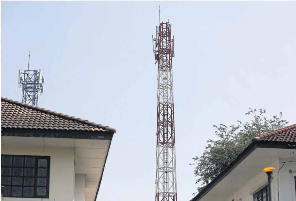
Telecom towers near a housing project in Bangkok's Sai Mai district. Concern has grown about the potential health ramifications of such towers.
