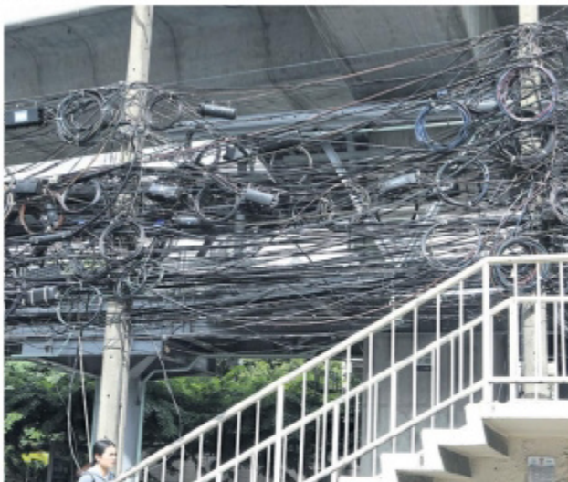
A rat's nest of cable wires hang above an overpass on Phahon Yothin Road in Bangkok. APICHT JINAKUL
